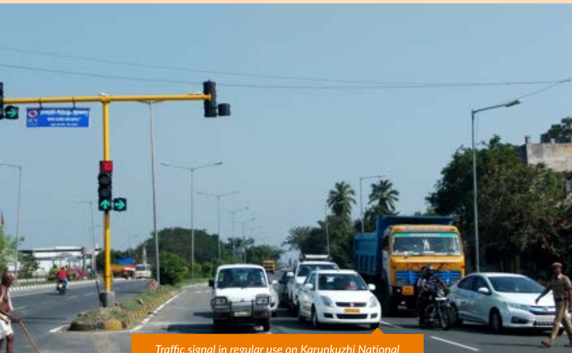
Traffic signal in regular use on Karunkuzhi National Highway in Maduranthakam (Tamil Nadu)
