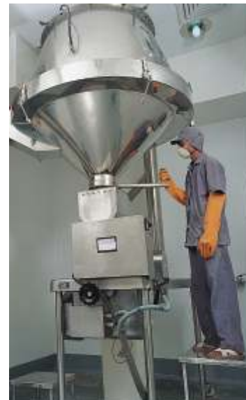
Gravity assisted material flow at the Silvas 2 plant
