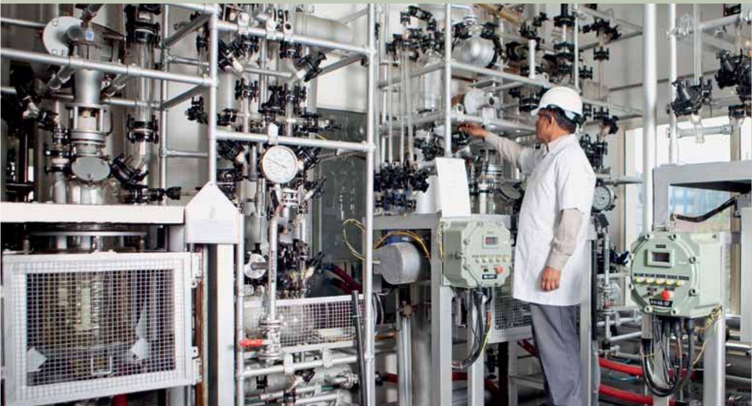
One-of-its-kind, the Triple Wall Glass reaction system for manufacturing high value products at the Ranbaxy Plant, Toansa, India
