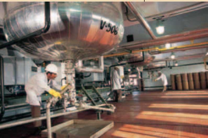
In the solvent recovery area, Ahmednagar
